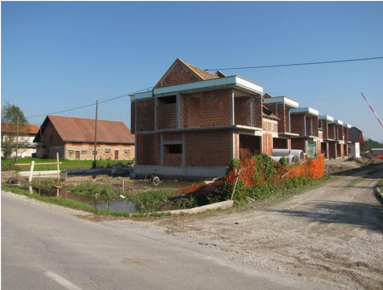
Flooding area as construction site
